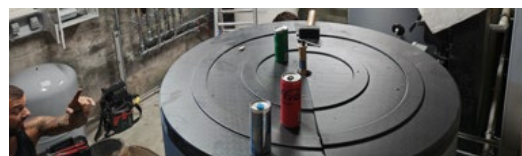
New battery and energy storage
