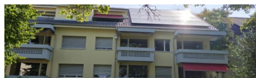
New photovoltaic system
